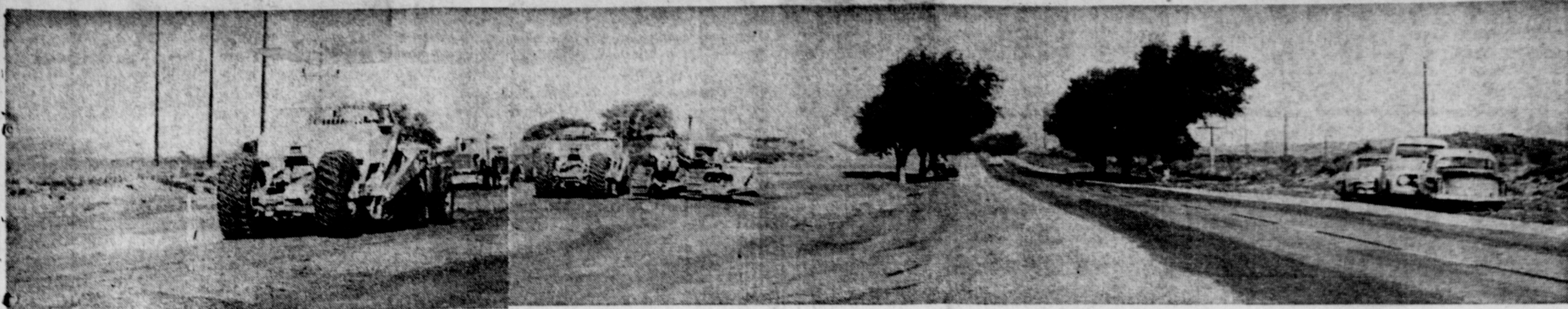
A W-I-D-E ROAD. The new four-lane highway east of Muleshoe on U. S. 84 will be this wide when completed. It will feature four lanes for traffic with a 67-foot division in the center. Work is moving rapidly on the project by Strain Brothers Construction Co. now (Journal Photo)
