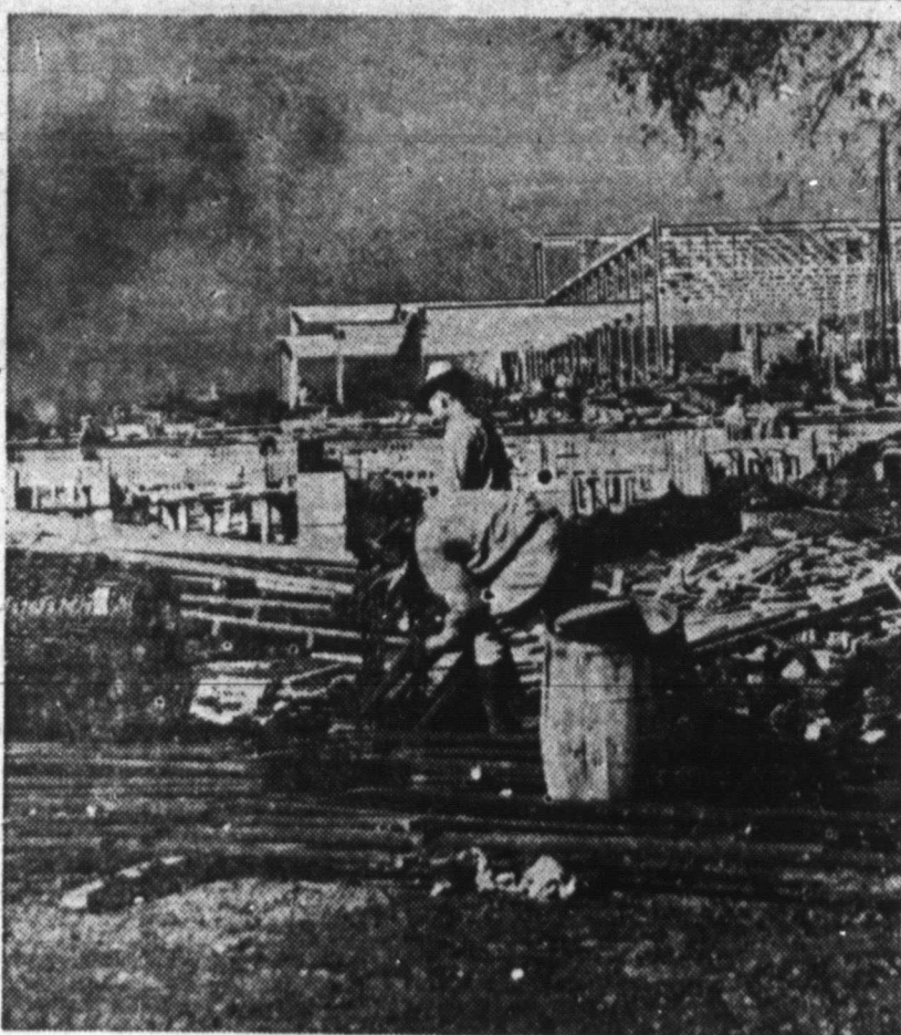
The steel frame of the $140,000 Livestock Building No. 2 for the Texas Centennial Exposition at Dallas can be seen above as it rapidly takes form. With the $250,000 Livestock Building
