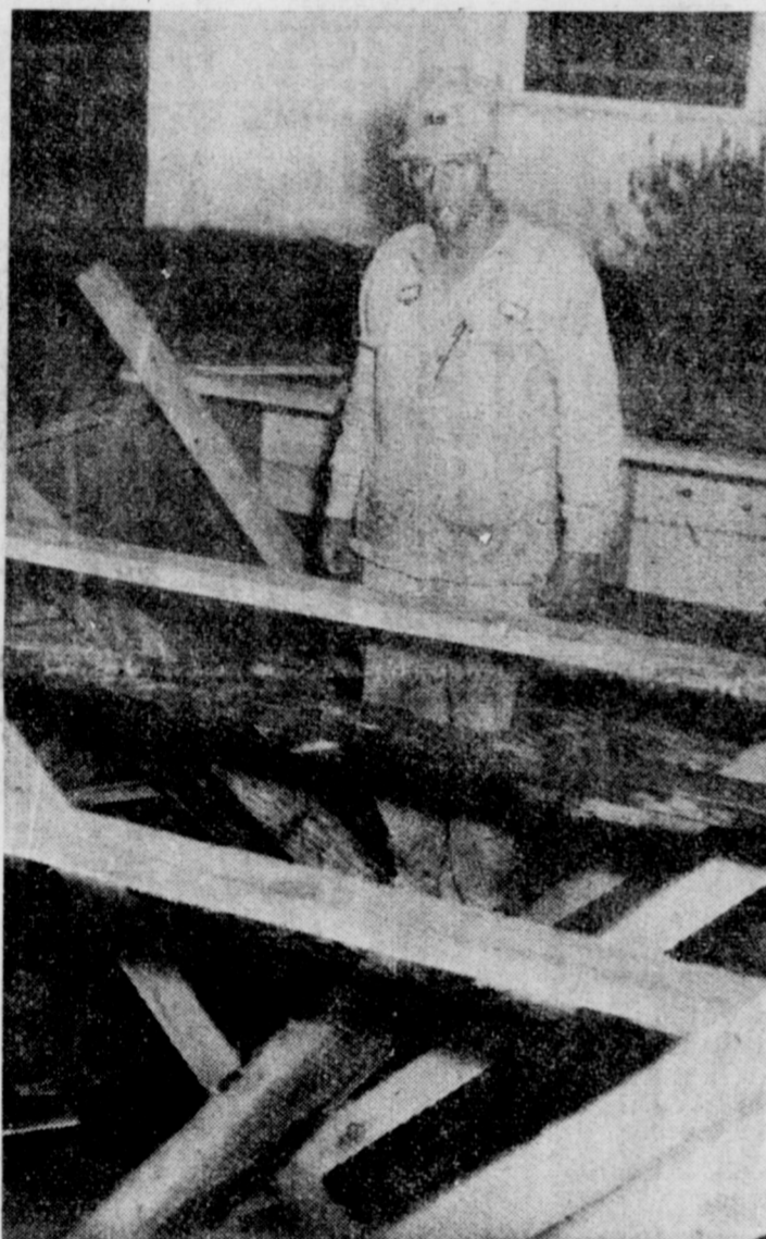
With the recent storm scares, a large number of local people are constructing storm shelters such as this one being built by Frank Mooney. (Staff Photo)
