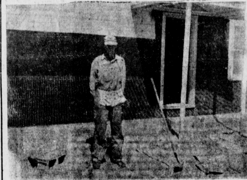
(Journal Photo) Home Sweet Home . . . C. C. Faulkner will soon be able to hang that sign in his new farm home eight miles east of Muleshoe. Faulkner is shown above in front of the four room house he and neighbors finished last week.
