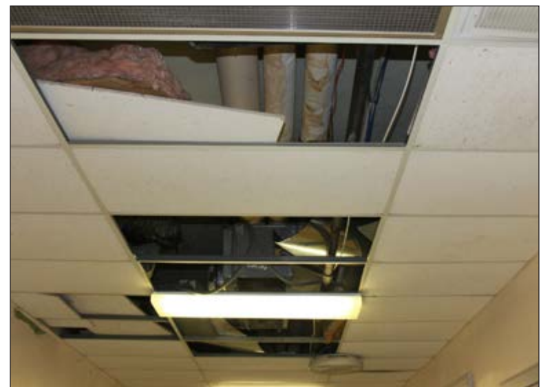
MELISSA PERNER | THE OZONA STOCKMAN MISSING CEILING TILES in the OHS Main Building expose insulation and conduit due to leaks. The CCCSD School Board discussed the building at the Nov. 14 regular meeting.
