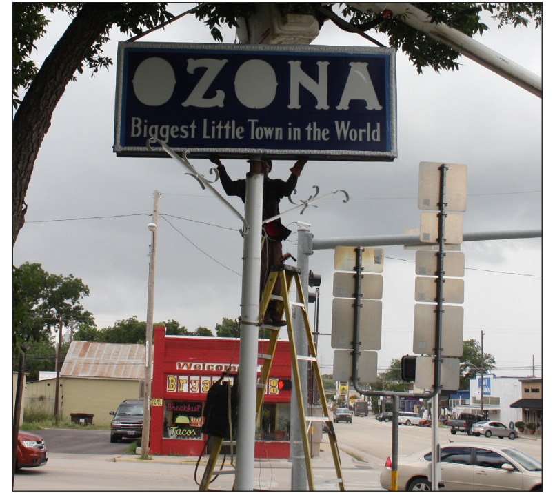
JOE HERNANDEZ | THE OZONA STOCKMAN THE OZONA SIGN in the town square got an upgrade. The new sign was installed last week and features new lighting and a more polished look. Crockett County paid for the sign renovations and employees of the county road department helped with the installation.
