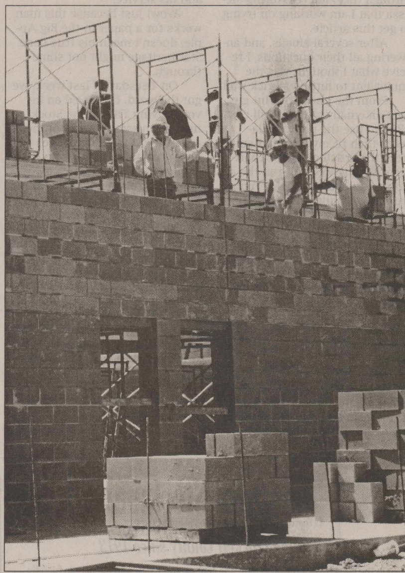
OZONA'S NEW ELEMENTARY SCHOOL is taking shape as workers start constructing walls at the site that once held the primary school. The school is scheduled to be completed by the start of the 2010-2011 school year.
