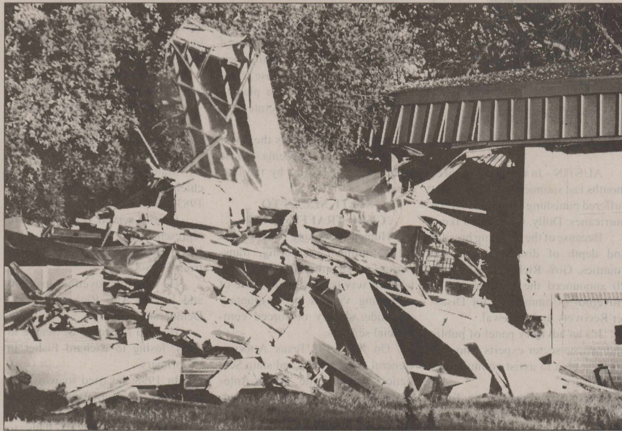
DEMOLITION WORK began last week at the Ozona Primary School Building. The school is being torn down to make way for the building of the new elementary school. The demolition is expected to take 4-6 weeks.
