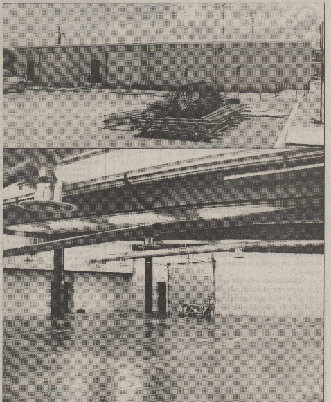
THE NEW FIELDHOUSE AT LION STADIUM is near completion. The bottom photo shows part of the roomy interior where the weight machines will be set up. DigiCam Photo by Scotty Moore
