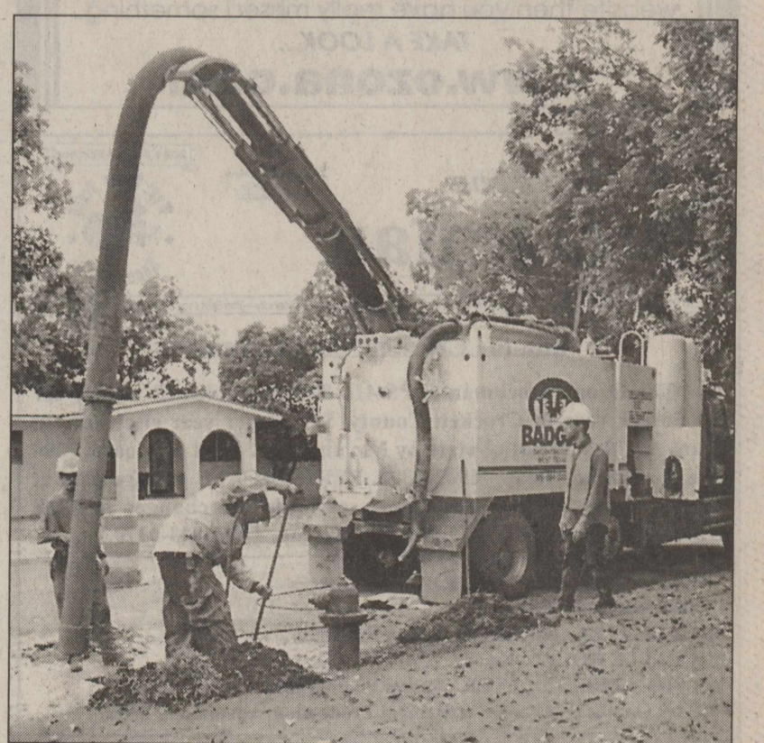
THIS HIGHLY SOPHISTICATED MACHINE uses high pressure water jets to dig around a hydrant while a vacuum hose removes mud and debris. DigiCam Photo by Susan Calloway
