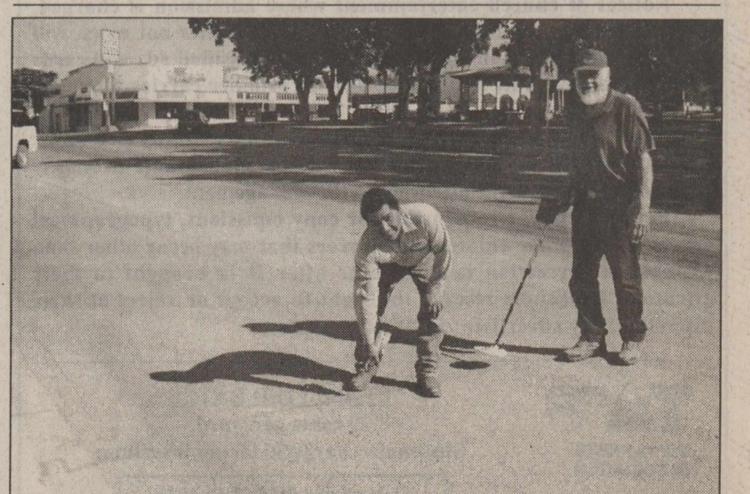
WATER DEPT. MANAGER DEE KEILERS uses a metal detector to find water pipes as Ricky Ramirez marks the pavement with spray paint. DigiCam Photo by Susan Calloway
