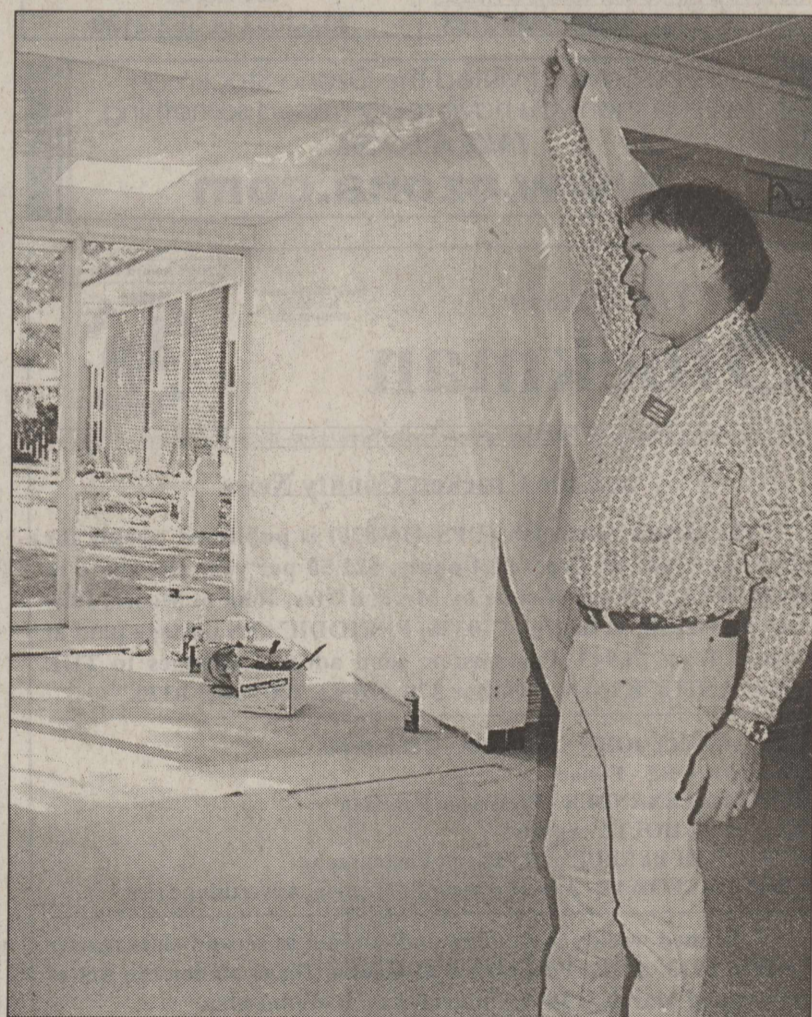
BENNY GIBBS, care center administrator, lifts a dust protector to show the enlarged dining area. DigiCam Photo by Linda Moore
