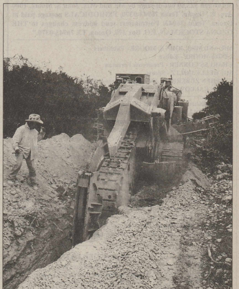
RISING DUST IS PART OF INSTALLING A WATER LINE to provide improved service to Crockett Heights and Circle Bar.
