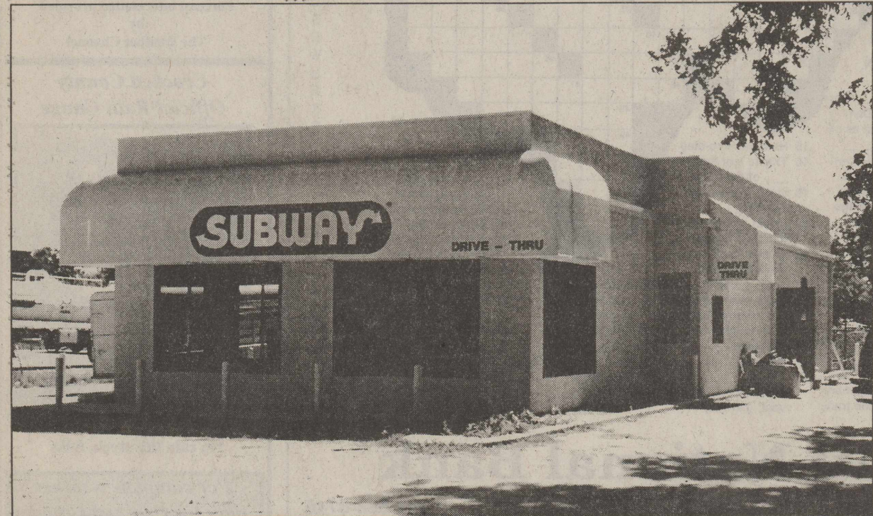
"UP SHE GOES"---Construction of Ozona's newest business, the Subway sandwich shop, owned by Shelly and Clay Childress is nearing completion and has been slated to open in the later part of July. The shop is being built between Town and Country Convenience Store and Crockett Automotive on Hwy. 163. DigiCam photo by Scotty Moore
