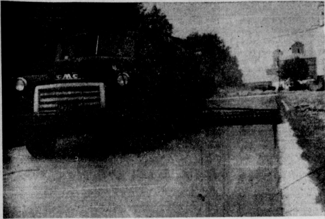
WORK IS ALMOST COMPLETE on the paving of 75 blocks of city streets in Muleshoe. Here a blacktop truck of Cen-Tex Paving Co. is laying a seal coat of hot topping on West Second street. (Staff Photo)
