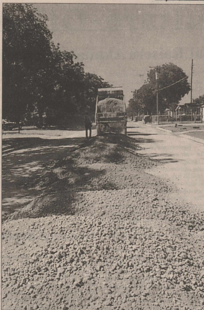
ROAD CONSTRUCTION on the 100 block of Ave. I continues this week. The paving will possibly be completed by Friday.
