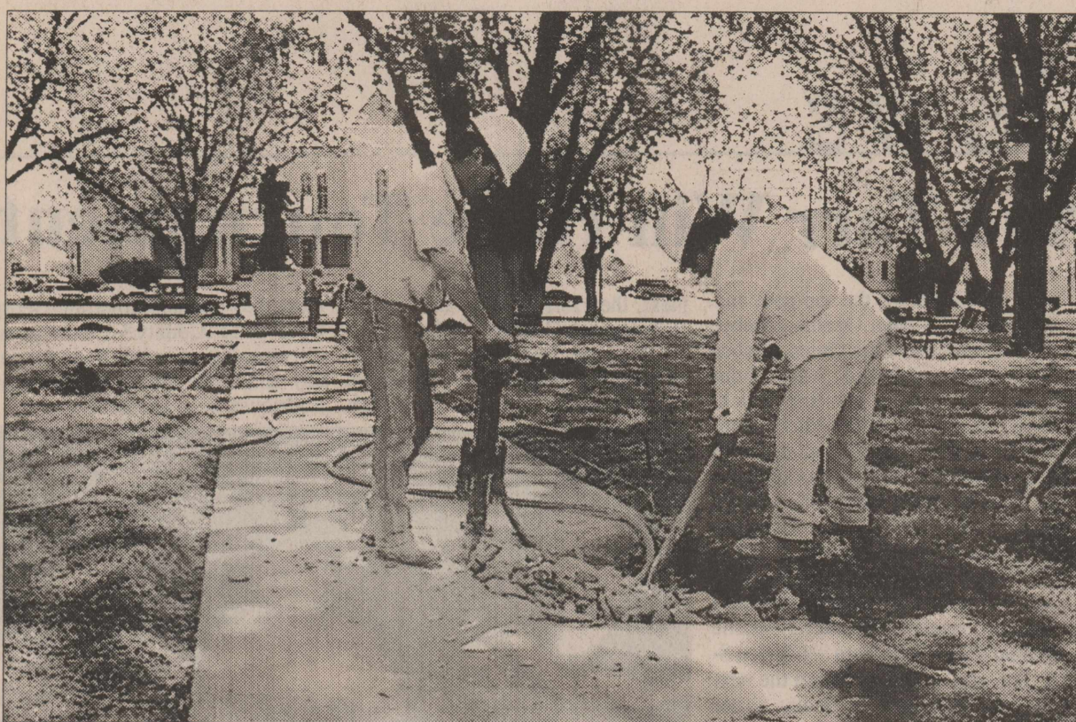
REMOVING OLD SIDEWALK on the square are Hector Garza and Miguel Rodriguez. Workers in the background are Juan Flores and Jaime Huerta. The sidewalk replacement project is a combined effort of Crockett County and Ozona Woman's Forum. DigiCam photo by Scotty Moore
