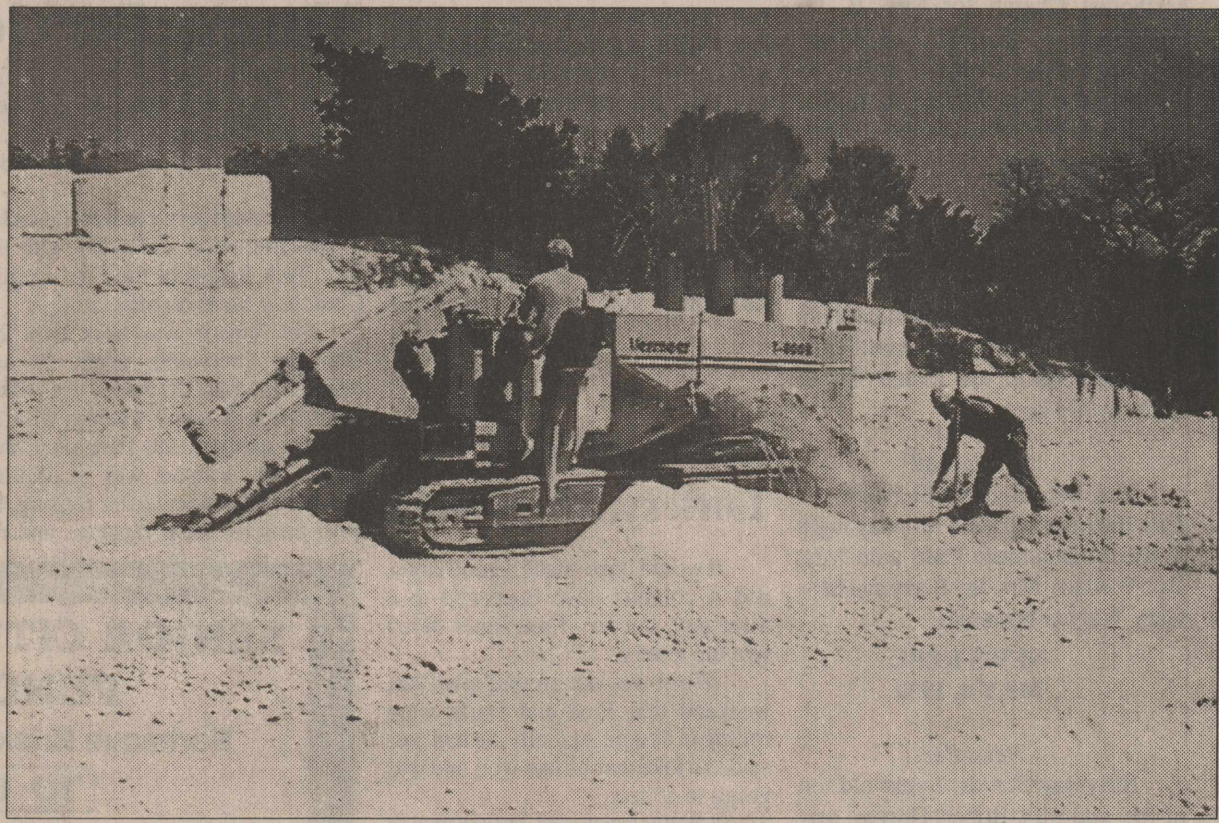
WORK STARTED last week in the area where the new courthouse annex will stand. An employee of Sundown Construction of Lubbock is digging the footing area to build the foundation. "Work is starting off real slow," said Eddie Moore, road and parks superintendent. "The next couple of weeks we will get something done."
