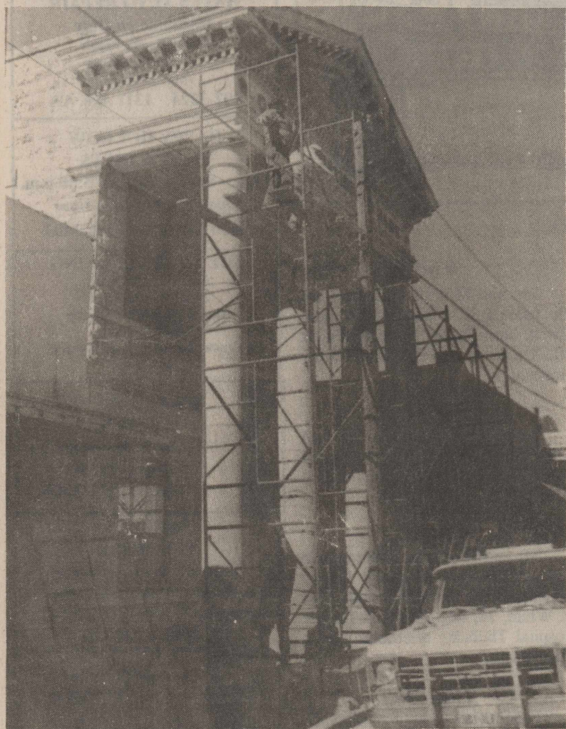
THE STATELY OLD OZONA BANK BUILDING, which houses the offices of attorney Bill Mason and CPAs Burl Myers and John Stokes, is prepared for painters to refurbish the trim. photo by Scotty Moore
