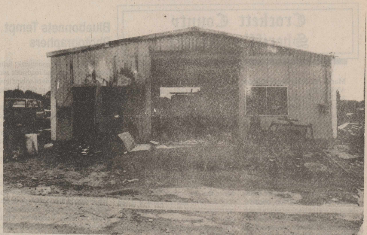
AN EARLY MORNING FIRE MONDAY gutted the office space area and overhead storage and John's Garage north of Ozona. Cleanup was underway later that day so the shop could return to business as usual.
