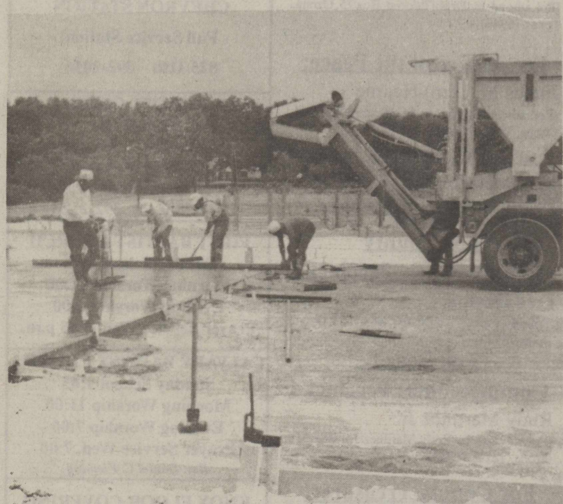
THE FIRST SECTION OF CONCRETE for the Fair Grounds Convention Center was poured Sept. 15 by employees of Lilly Construction Company. This portion of the $300,000 project is expected to be complete by Sept. 23 and work on the structure will begin next week.
