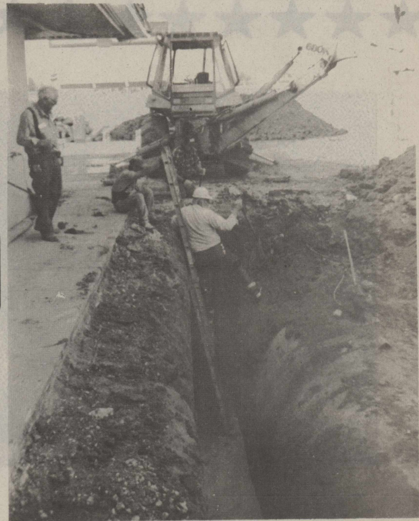
WATER DISTRICT MANAGER DEE KEILERS inspects and repairs the broken sewer main that was accidentally perforated Monday by a back hoe at Shots #4 south of Interstate 10. A contract company was in the process of digging up and replacing the underground storage gasoline tank at the store when it accidentally hit the sewer line.
