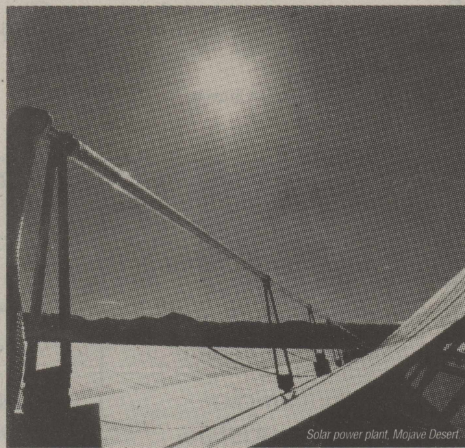
Solar power plant, Mojave Desert.
