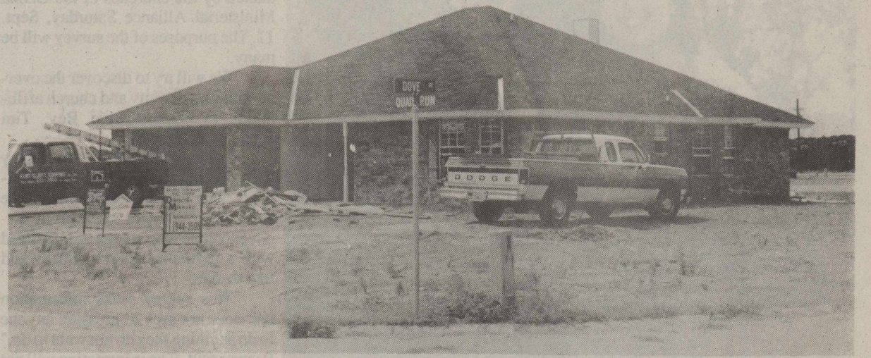
CONSTRUCTION AT 102 QUAIL RUN is in the intermediate stage, the brick is on and sheetrock is in. The properties are handled Doris Thieman of Dierschke Mikeska Realtors.
