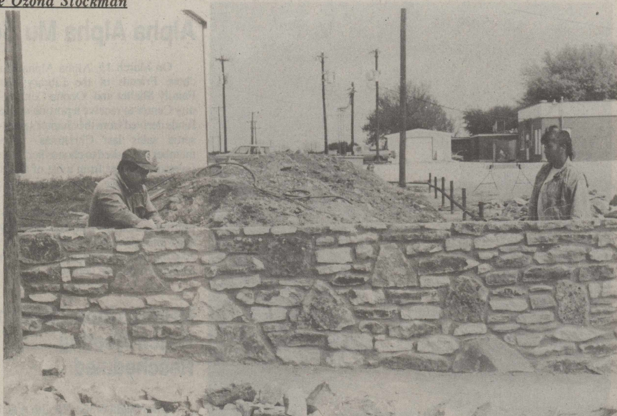
CLARO AND MARIA QUIROZ were busy Saturday working on a rock retaining wall at the new EMS building. Quiroz has been an independent stone mason since 1985 after years of working with others.
