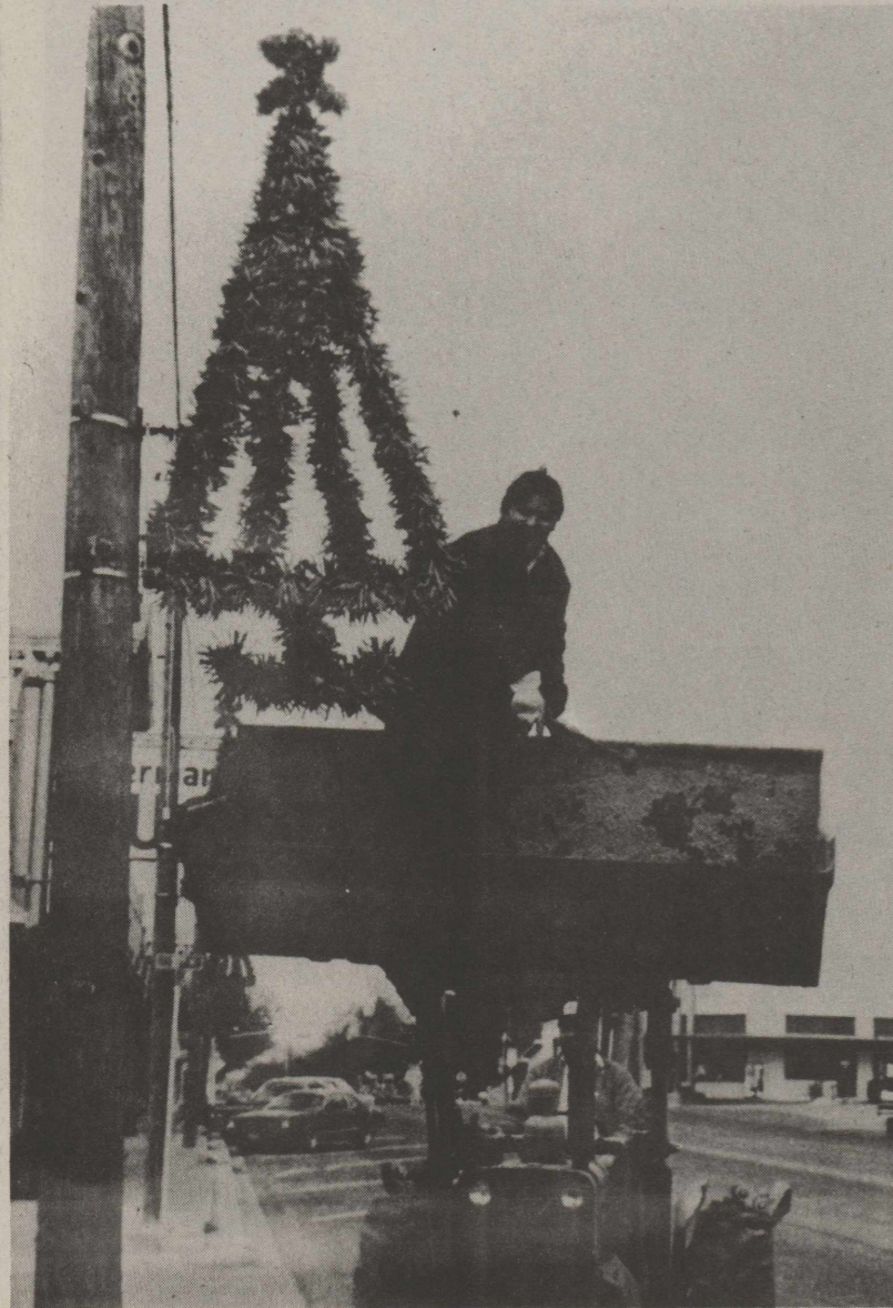
HELPING OZONA GET INTO THE CHRISTMAS SPIRIT are Crockett County Water District employees Ricky Ramirez (in bucket) and Alex Borrego.
