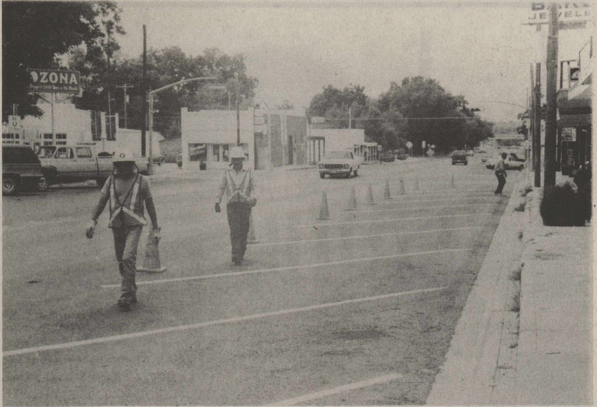
TEXAS DEPARTMENT OF TRANSPORTATION EMPLOYEES place warning cones along the square during re-painting of the parking lines.
