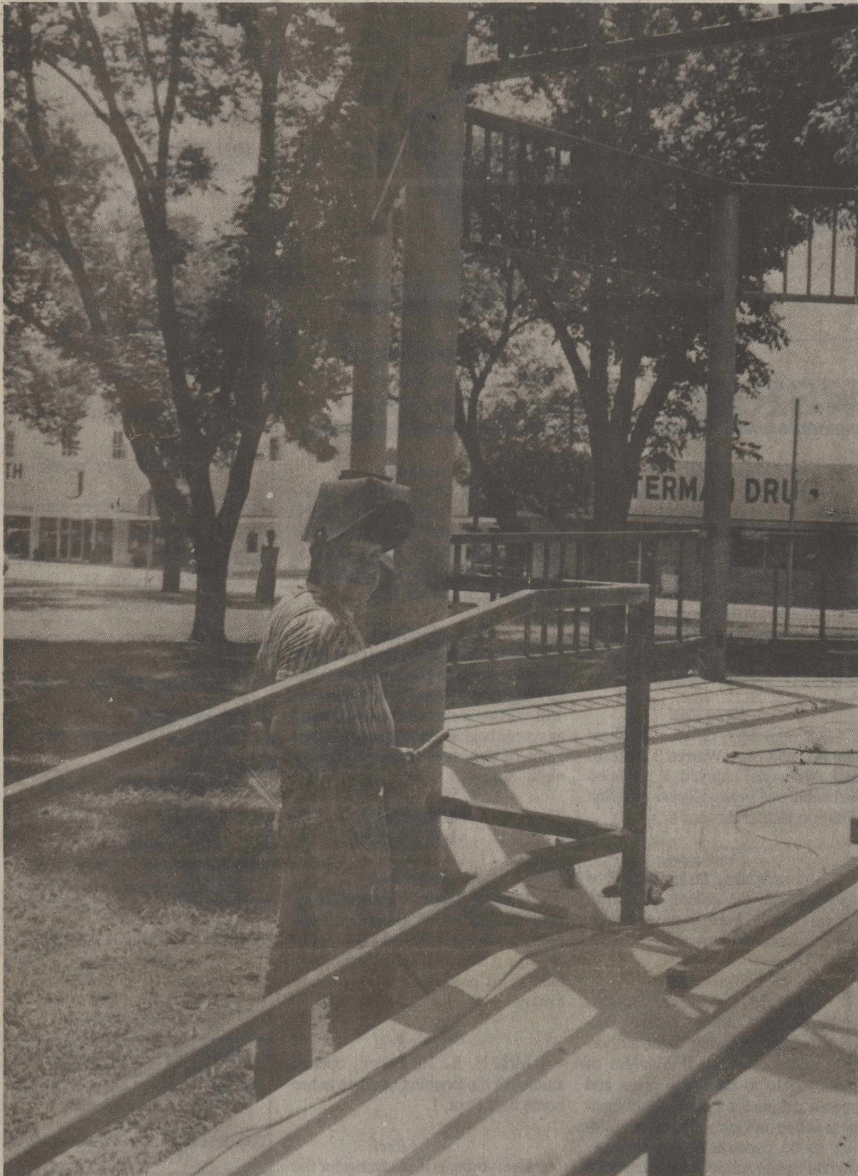
ALEJOS LARA has been hard at work lately building the metal railing and roof support structure for the new bandstand in the park. Alejos has donated his labor and expertise in the construction of the new stand.
