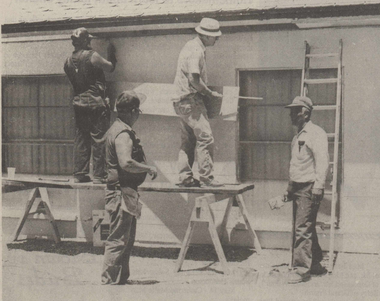
Workers from area churches were in Ozona Saturday to help with repairs and painting at Calvary Baptist Church. Pictured are Steve Mobbs, George Hester, Ted Dews and Rosalio Longoria.
