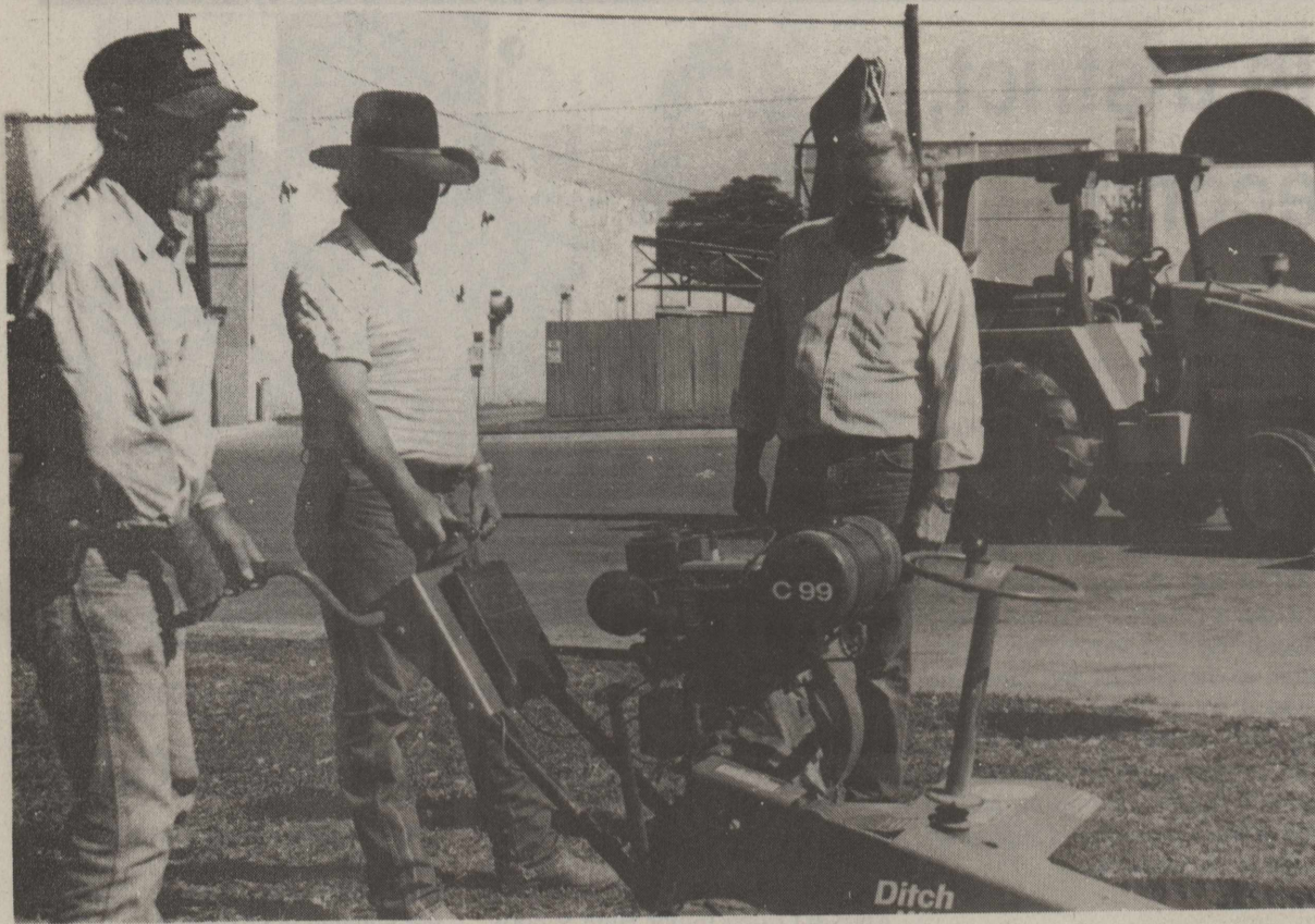
Preparing to begin work on the sprinkler system on the square last Friday are: (l. to r.) Johnny McCary, Eddie Moore, J.C. Schroeder and David Tijerina (on tractor).
