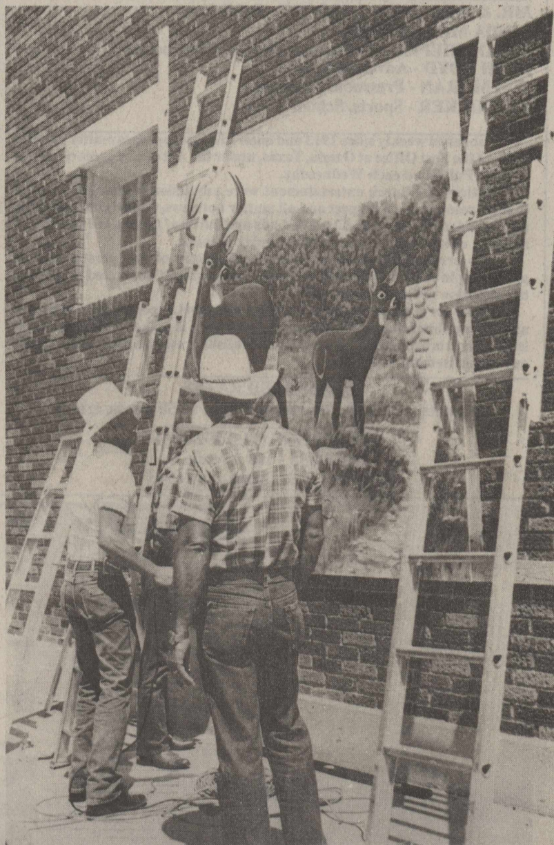
Artist Jack Feagan (left) and his brothers Jerry and John install the first mural on the Perner Building August 11. This mural, paid for by the Ozona Chamber of Commerce, will be joined in two weeks by a second made possible through donations.
