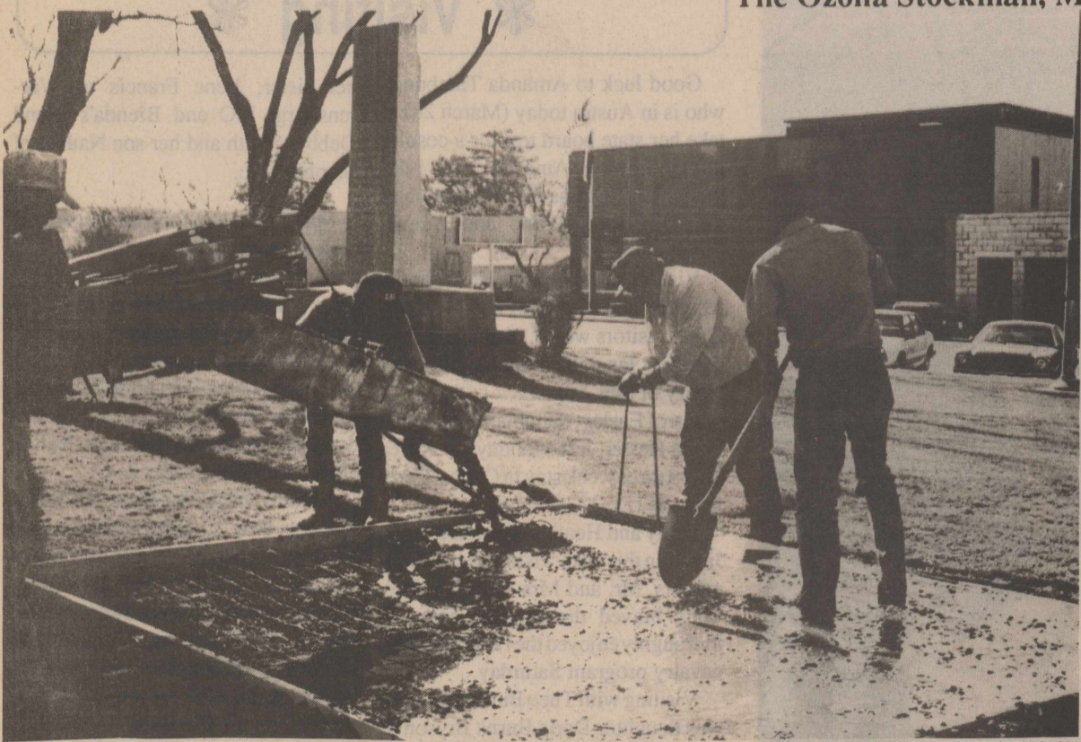
County workers busily prepare the foundations for the picnic tables on the square. This project is a joint effort of the Ozona Chamber of Commerce, Crockett County and the Texas Parks Department to encourage visitors to stop in Ozona and see what our fine town has to offer.
