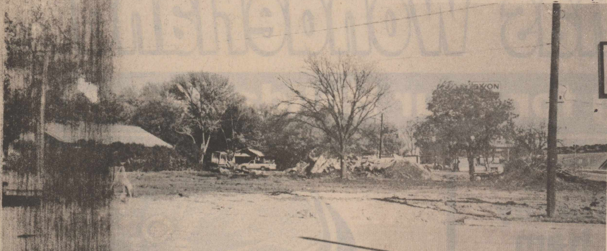
The new Dairy Queen is expected to be completed in March as work continues this week to clear these lots on Avenue C. by I-10.
