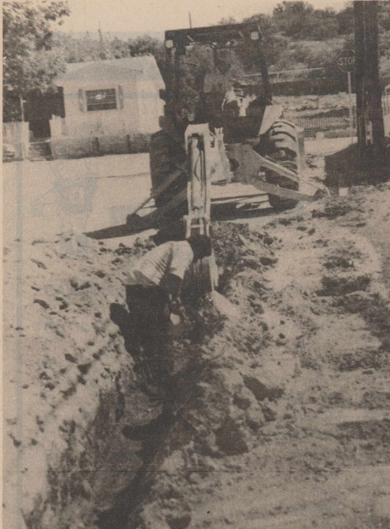
Ozona water control employees work on Santa Rosa St. checking water lines before county road workers resurface the streets. Work to relieve drainage problems in this area continues this week.
