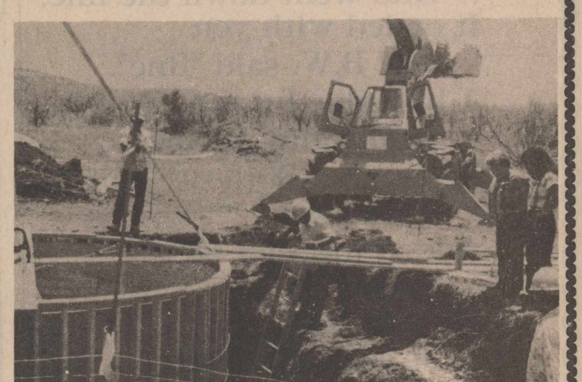
Pump station construction being examined by water district employees Alena Faye Hokit and Ampara Enriquez.
