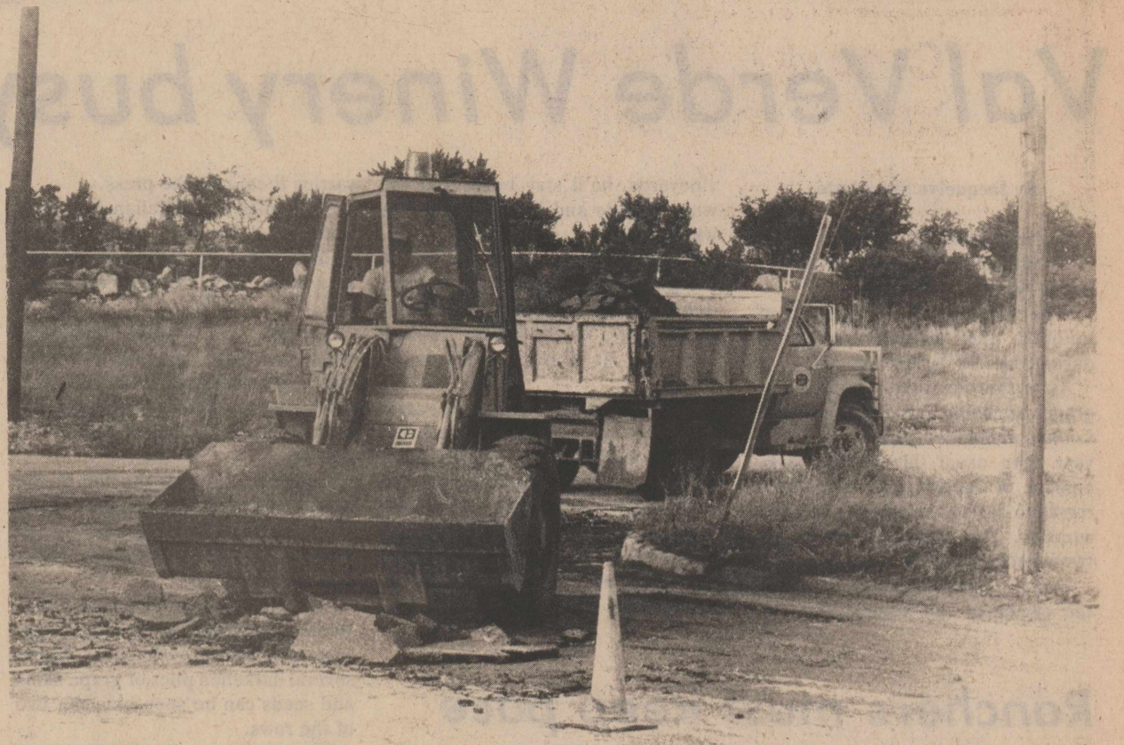
Richard Sanchez is busy cleaning up pavement damaged by four plus inches of rain Aug. 13. This section of Ave. J turned into a narrow, one-lane street until repairs could be made. Assisting with the cleanup were Albert Borrego and David Tijerina. Photo by Linda Moore
