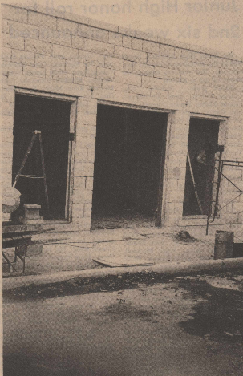
RENOVATION BEGINS at the old Davidson building next to Ozona National Bank which housed the Ozona Stockman for fifty years. The building, which had fallen into disrepair recently received a new roof and the rock facade, which had been painted, has been sandblasted.
