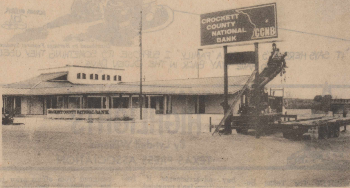
New sign for CC National Bank. Workmen were busy last week putting up the new sign at Ozona's newest bank. The lighted sign will have the time and temperature.
