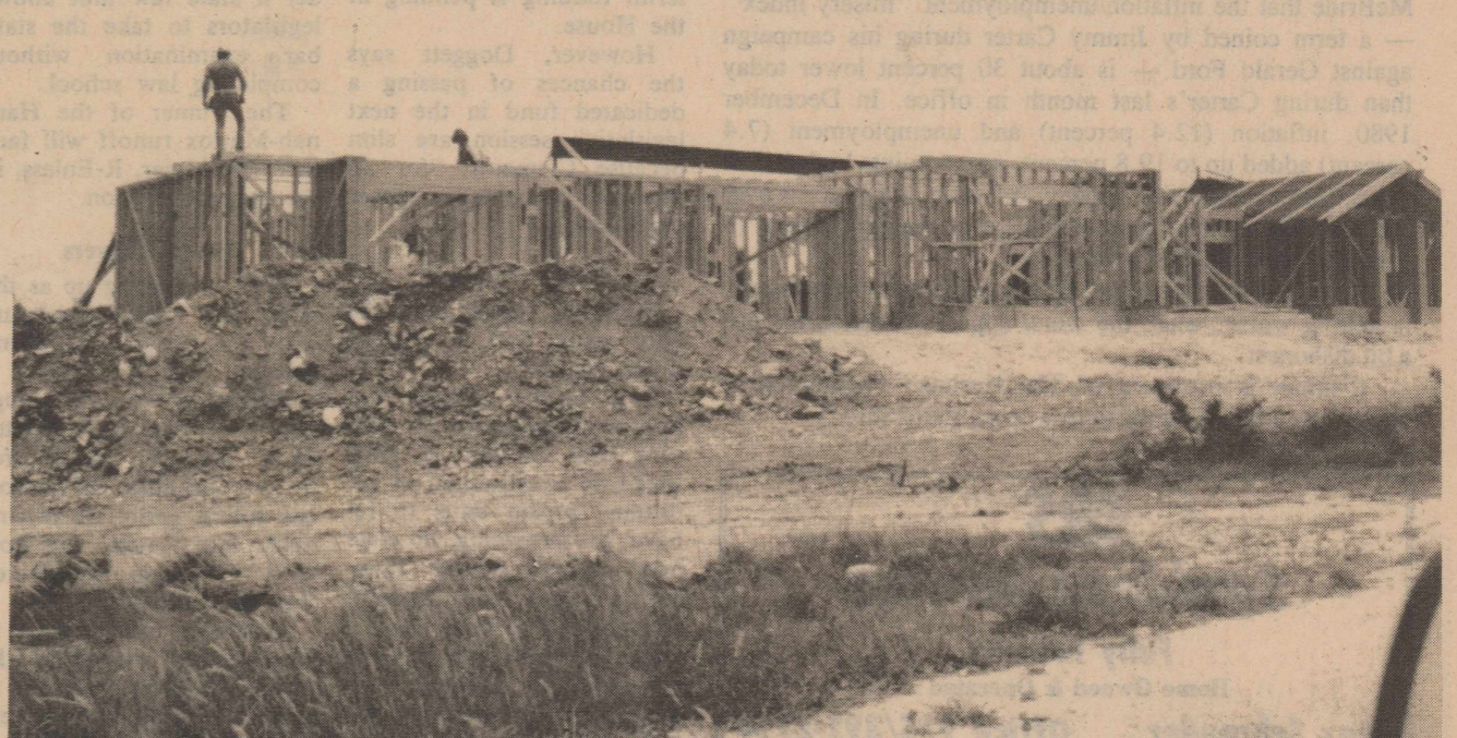
UNDER CONSTRUCTION on the west hill is the new home of the Tom Camerons. The Steve Sessom home is going up in Country Club Estates, and the Pon Seahorns are
