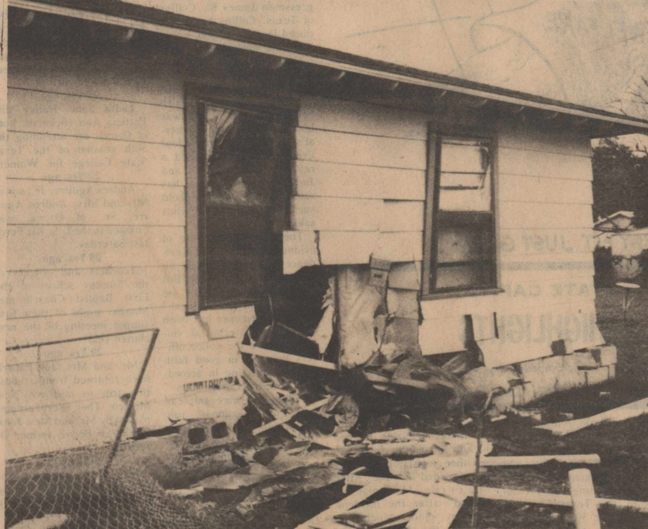
TRUCK CRASHES INTO HOUSE-This was the scene Tuesday morning at the Flores home where a truck crashed into the north side of it late Monday night. Both bedrooms in
