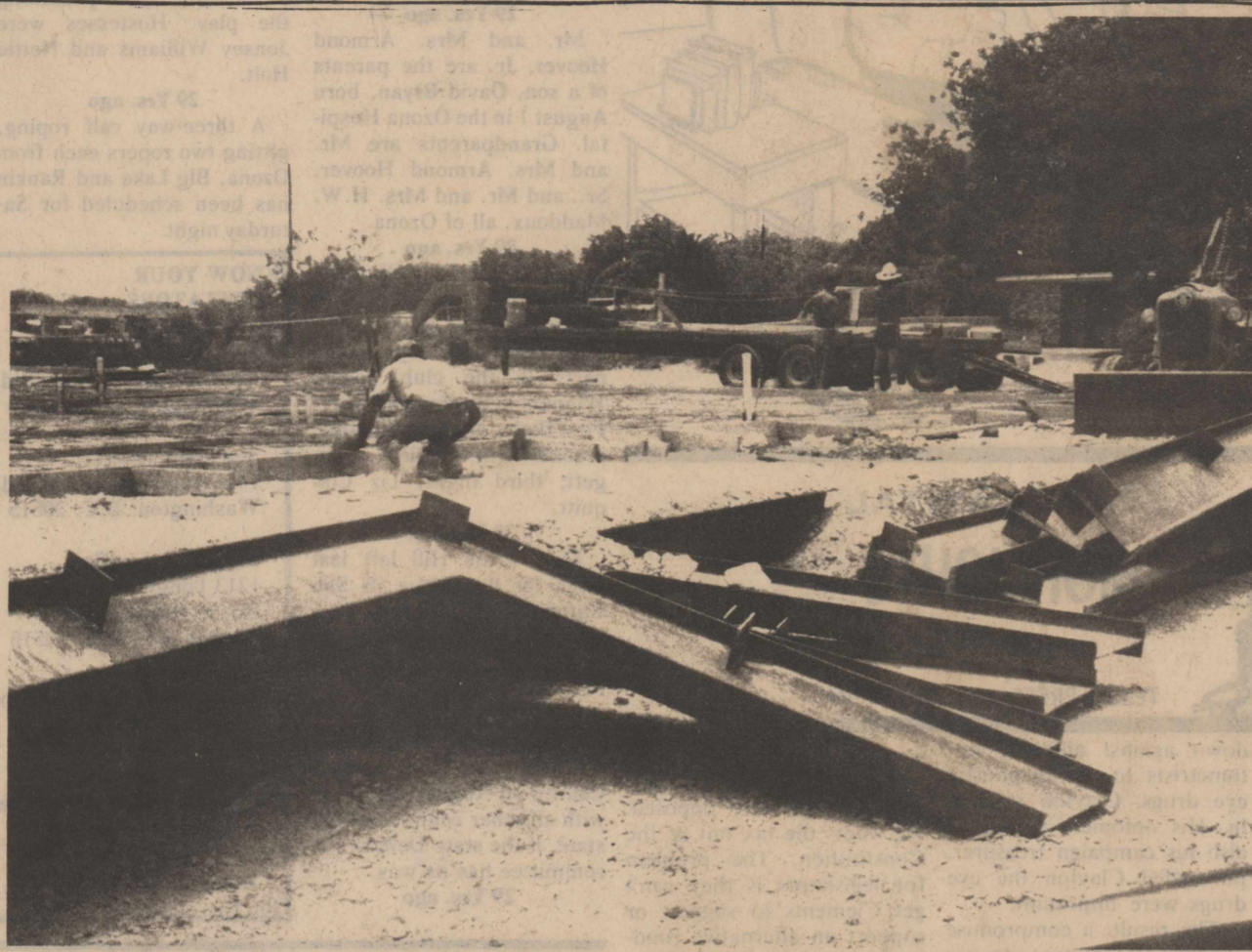
NEW CONSTRUCTION FOR OZONA-The foundation is being laid for a new 12-unit office building on Johnson Draw near the Inn of the West. The building, a project of Charles Williams, John Childress and D. E. Jackson, will be steel and glass construction with a brick or rock front. Completion date is projected for October 1.
