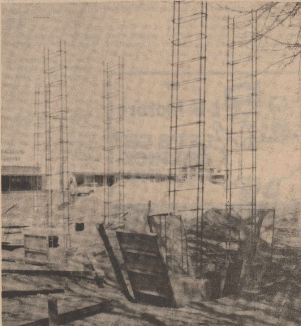
CONSTRUCTION BEGINS on Ozona National Bank's new drive-in facility across from Foxworth-Galbraith on Ave. E. What looks like several tall steel ladders is actually the beginning of the modern new drive-in bank. Weather has been perfect for construction, and if it continues, the building will be finished in record time.
