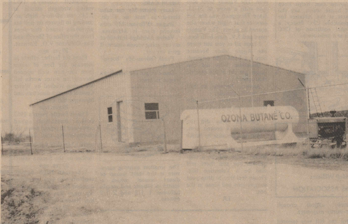
NEW PLANT UNDER CONSTRUCTION-Future home of Ozona Butane Co. is located across from the cemetery on Hwy 163. The large steel building will house the offices and all facilities presently located in the downtown building and
