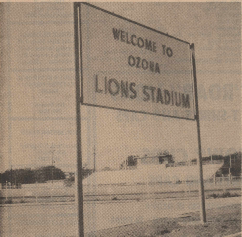
NEW SIGN WELCOMES visitors to Lion Stadium. The sign was made by Karl Vancil's vocational agriculture classes and installed Friday at the stadium at the north end. The gold sign with purple letters carries out the Ozona school colors.
