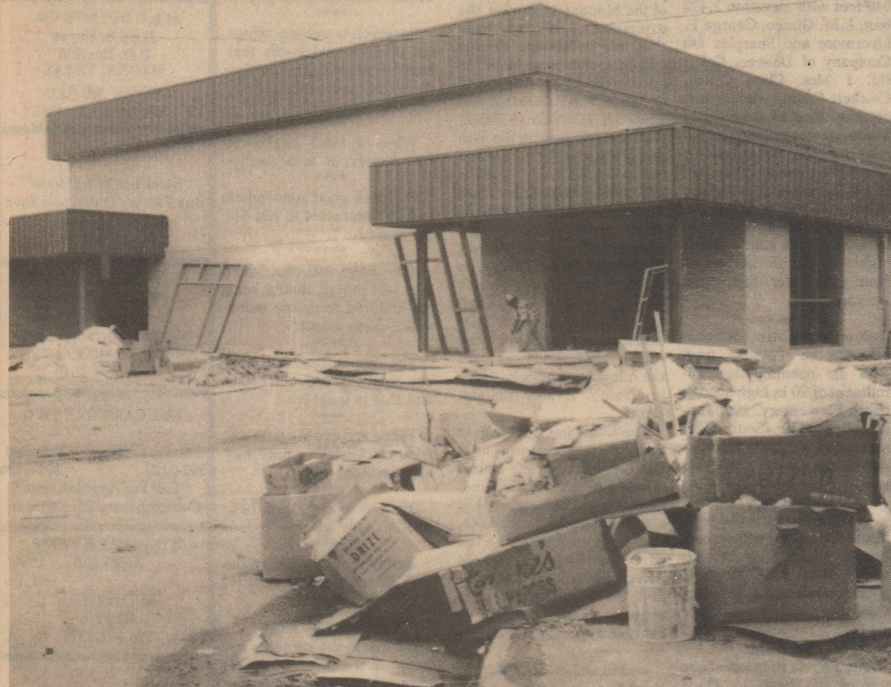
SCHOOL CONSTRUCTION was so far behind when time came for the opening of the fall term Tuesday that the school board thought it in the best interest of the school system to postpone the opening until next Monday, Sept. 11. The debris in front of the junior high gymnasium is typical of the conditions the board found in its inspection Monday. However, it was the conditions inside the buildings that caused the postponement.
