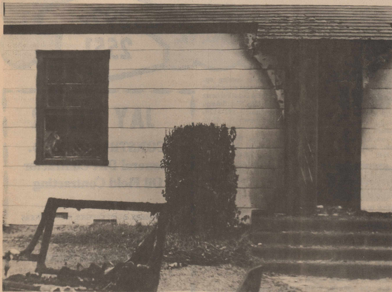
FAST SPREADING FIRE DEMOLISHED THE INSIDE of the Fred Buie home on Beall Street Saturday night. Although the home was occupied, the fire discovered immediately and firemen called to the scene in a matter of
