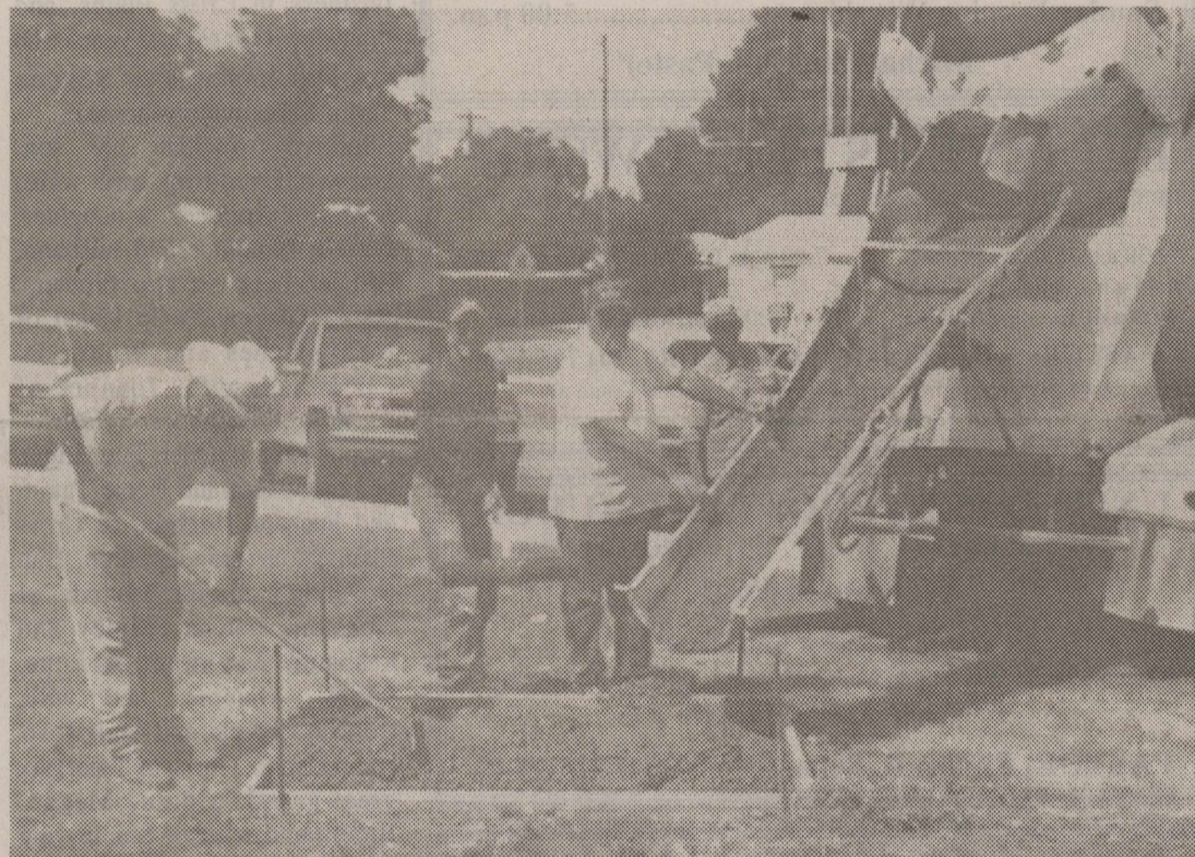
SCHOOL PRIDE LIVES ON —Fond memories are precious to all of us. Even with a heavy work schedule Reed Construction made time to donate the labor and materials for the concrete slab for the buffalo. Assisting with the project were Rusty Reed (class of 1971), Robert Bennett (class of 1974), and Cody Reed (class of 2001).
