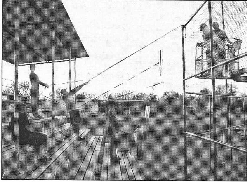
EAGLE PROJECT —Haskell Boy Scout Troop 136 assisted Scout Tucker McCormick with his Eagle project finished last May. McCormick's group painted the fences and replaced the wire mesh on the posts at the Little League park. Hoisting the fencing material up the fence posts while the men in the manlift fasten the wire to the posts are, l-r, Daniel Contreras, James Bowers, Tyler Reese, Lance Sloan and in the manlift are Chris Shelton and Craig McCormick.
