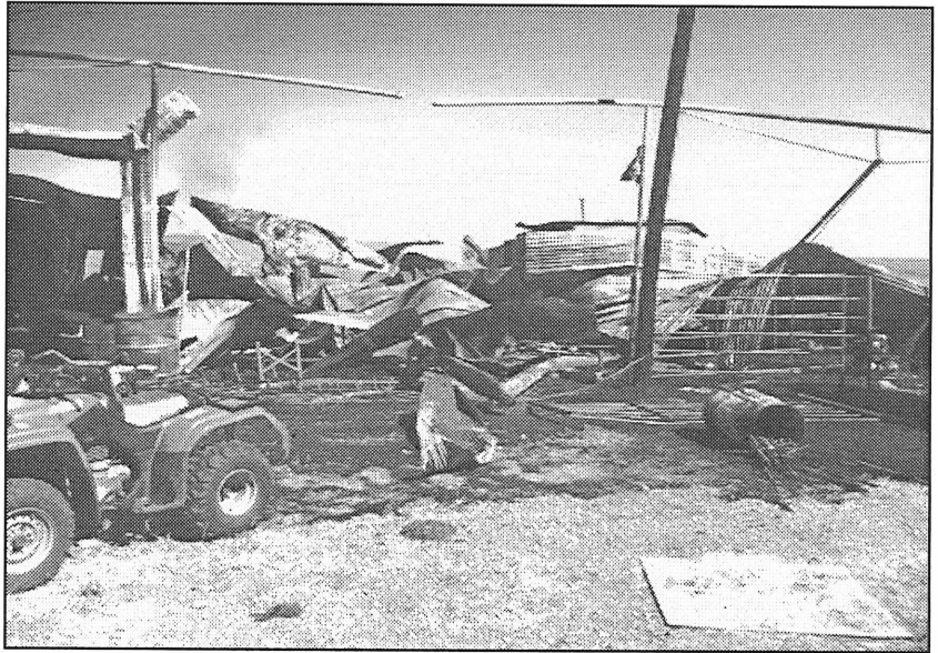
BARN FIRE —Haskell volunteer firemen responded to a barn fire Thursday morning Oct. 9 just before noon. The barn, belonging to Fritz Buerger, was located about six miles north of Haskell on FM 2163. Contents and the structure suffered severe fire damage.
