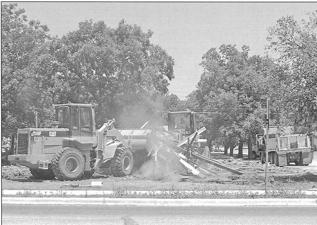
CLEANUP FOR SAFETY —Cleaning up the site of the old library building, which is being razed in readiness for construction of a new Haskell County Library, crews were busy Monday, clearing debris for the safety of children playing and for mowing purposes. Those helping were crews and machinery from County Precincts 2, 3 and 4, and the Community Service Workers Department.
