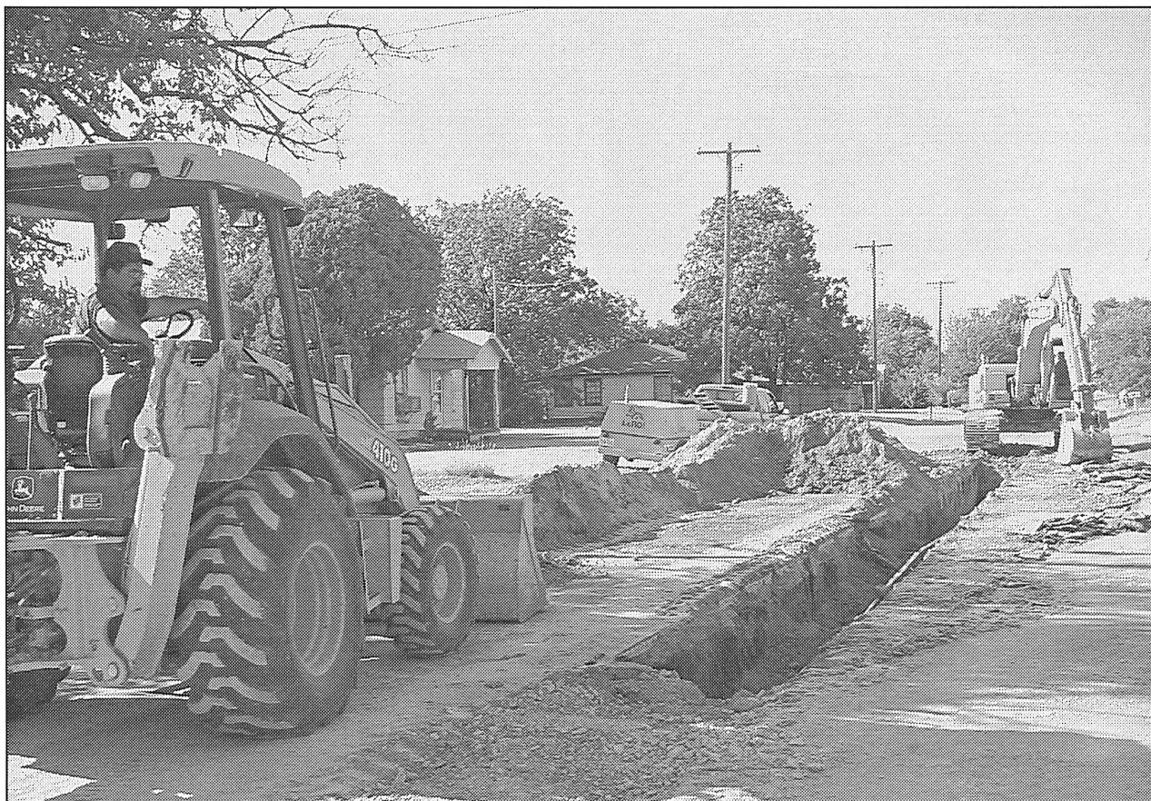
REPLACING WATER LINE—Employees of Tec Excavation of Midland, were busy Monday, working on the completion of a new waterline
