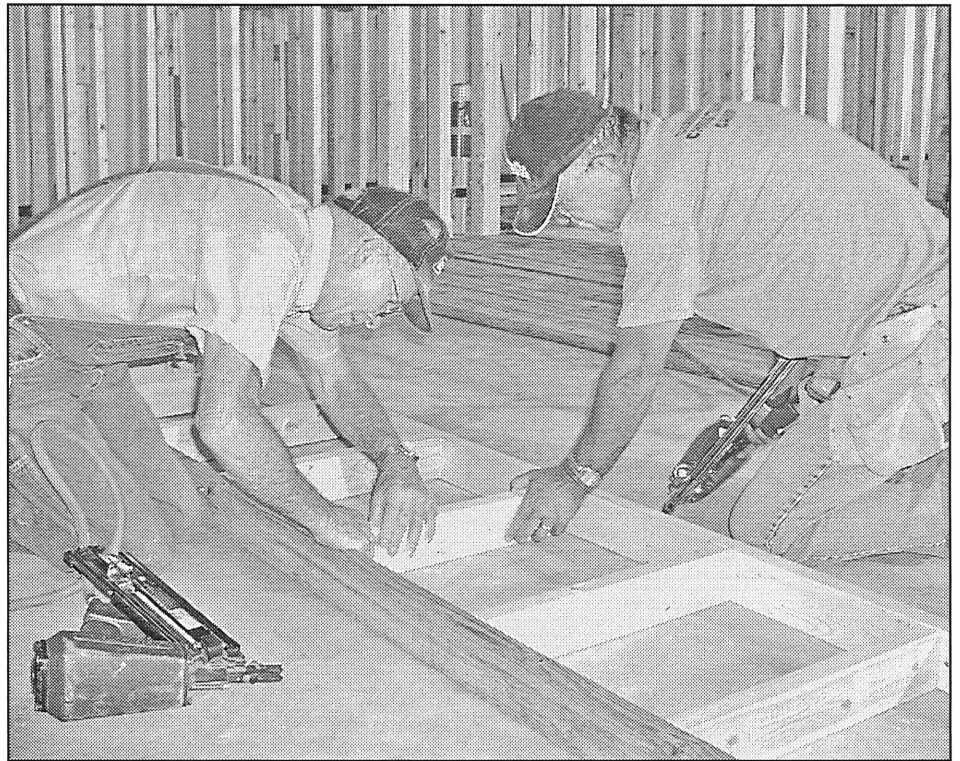
HELPING HANDS —Wayne Wainscott of Haskell, left, assists John Taylor of Odessa, in preparing support structures for the platform in the new sanctuary of Cornerstone Fellowship Baptist Church.
