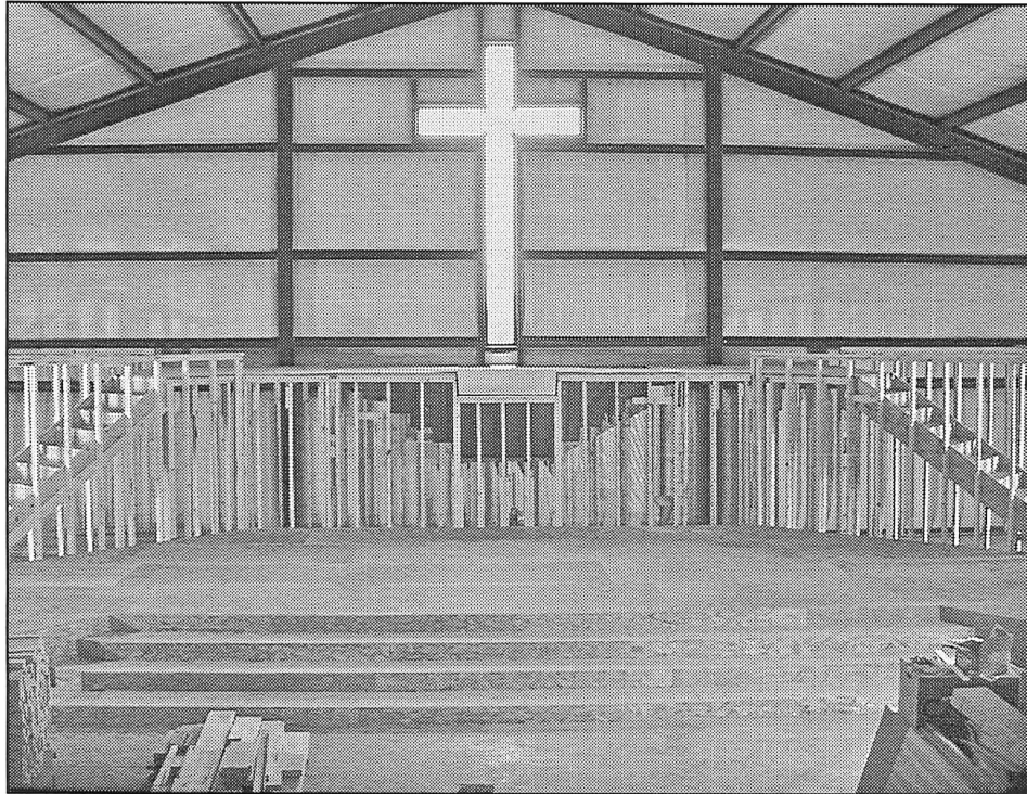
FRAMING THE WORSHIP CENTER —Aided by a group of 13 volunteers from Texas Baptist Builders, who are associated with the Southern Baptists of Texas Convention, local workers continued to raise and finish the platform in the new sanctuary of Cornerstone Fellowship Baptist Church.
